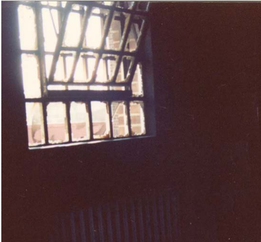
Melted glass windows.
