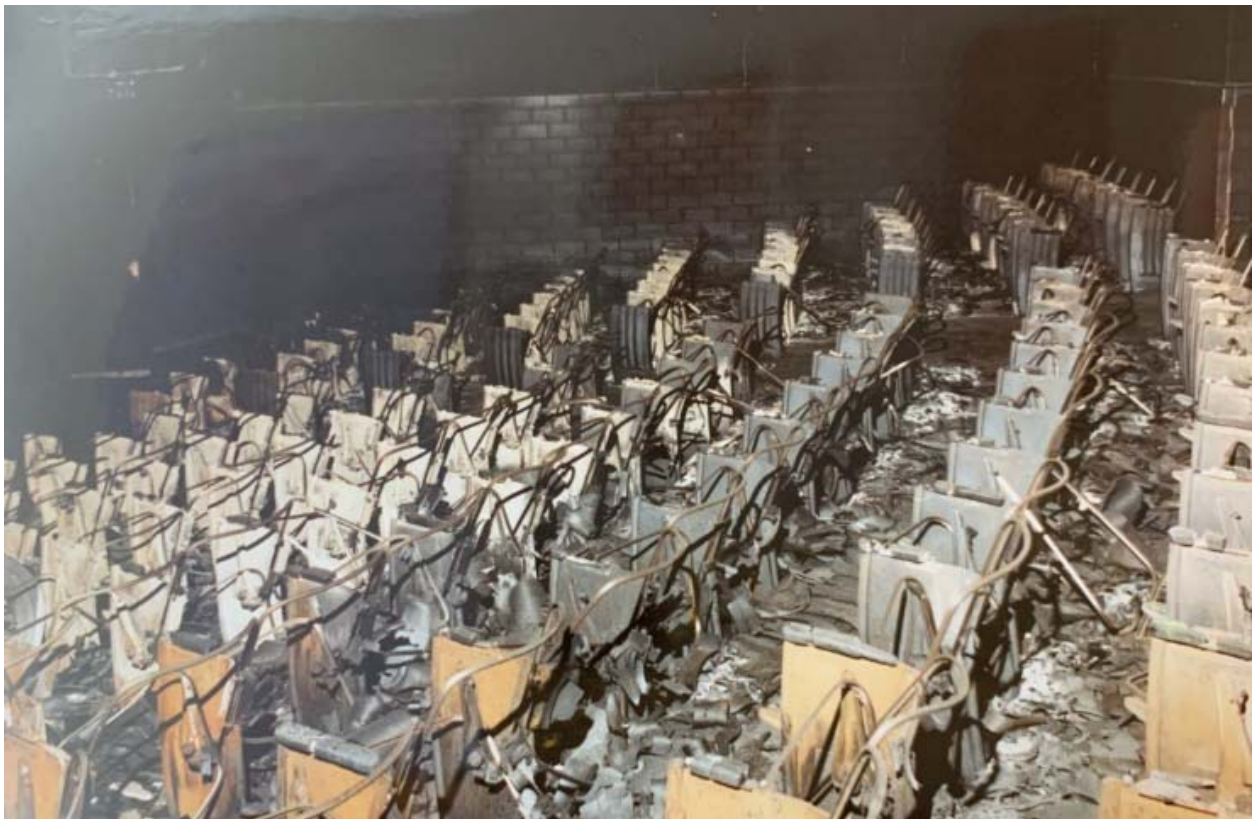
The destroyed auditorium.
