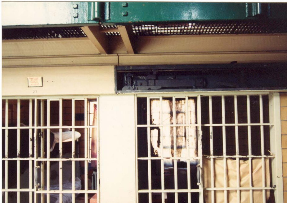
This picture shows the control area above the cell doors. The switchbox, not shown, is what controlled these levers to open or close cell doors.
